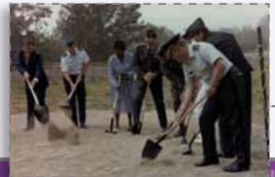
DoD invests $100 million into construction of new facilities on Presidio of Monterey. Col. David Mc Nerney (far right) breaks ground on Nicholson Hall in 1985
